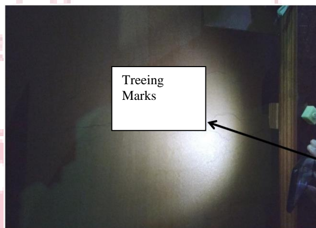
Fig. 3.6 Treeing marks outer surface of outer most pressboard barrier of U-phase coil
